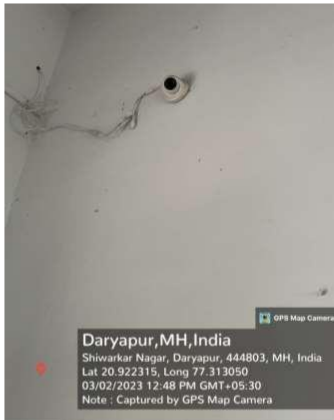
CCTV Camera in Classroom
